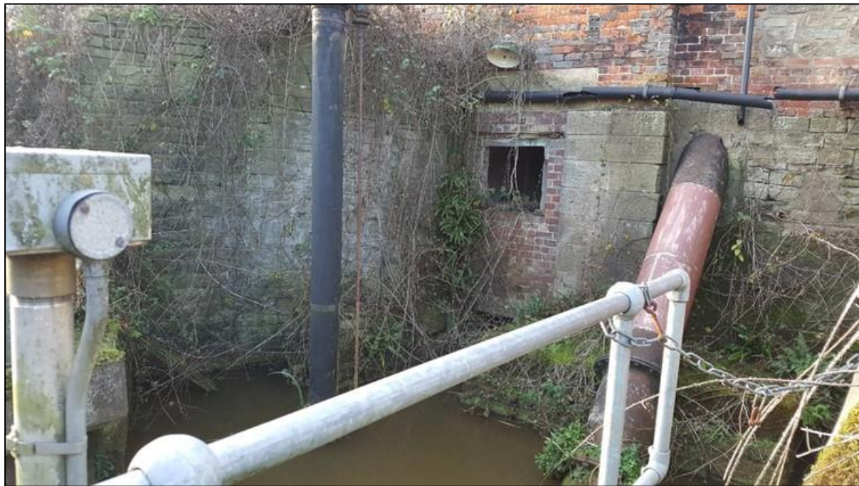
Figure 3-6 Holmeswood Pumping Station
